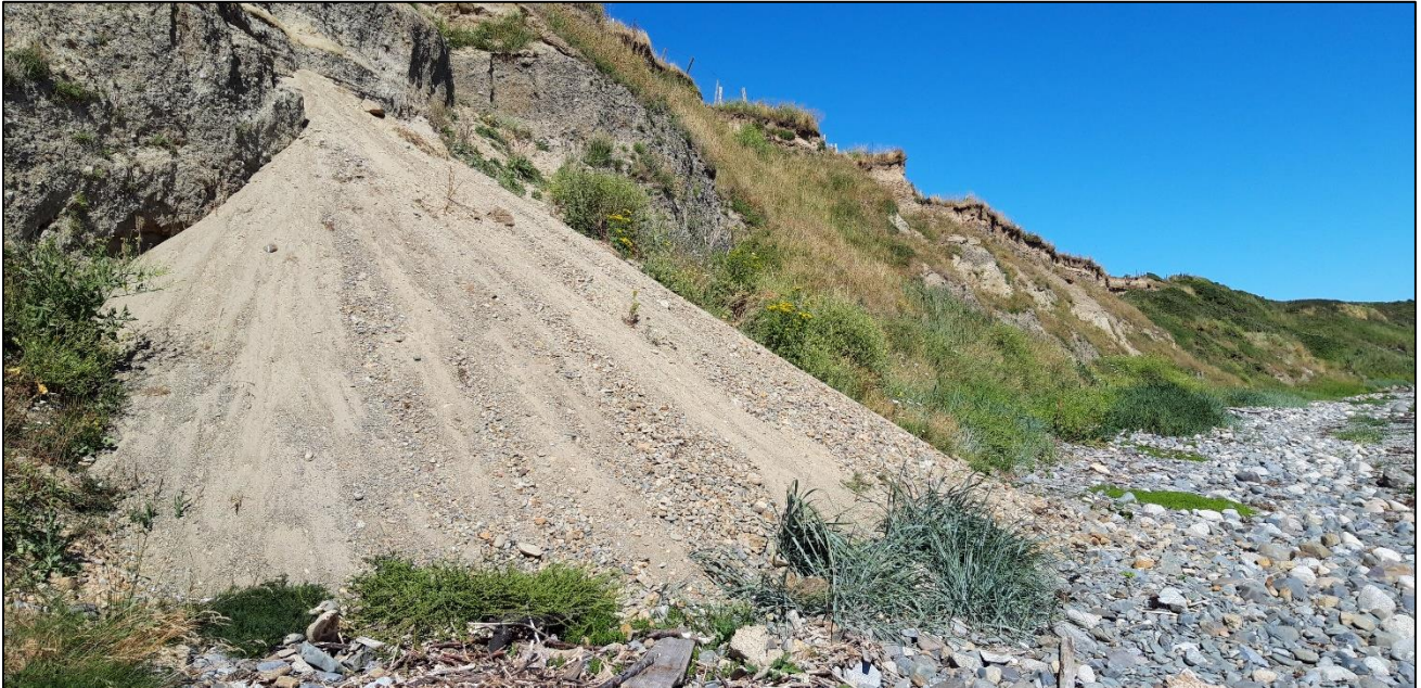
Figure 3.3. Recent erosion on a section of cliff.
